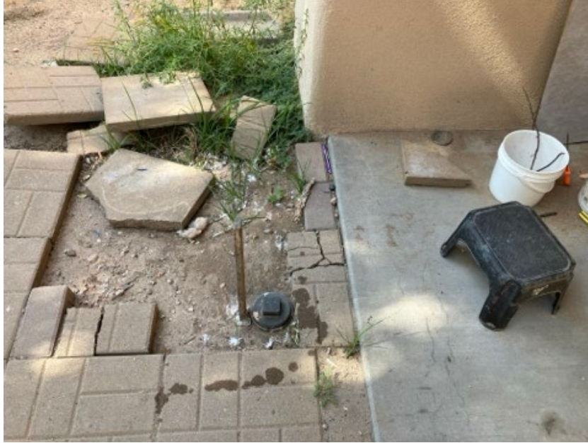
View of the existing sewer service line (SSL) cleanout at the south wall of the house. The new SSL will connect to the house at the same location.
