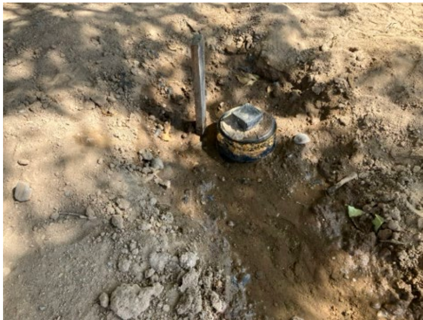
View of the cleanout at the existing septic tank. The existing tank will be crushed and abandoned in-place.
