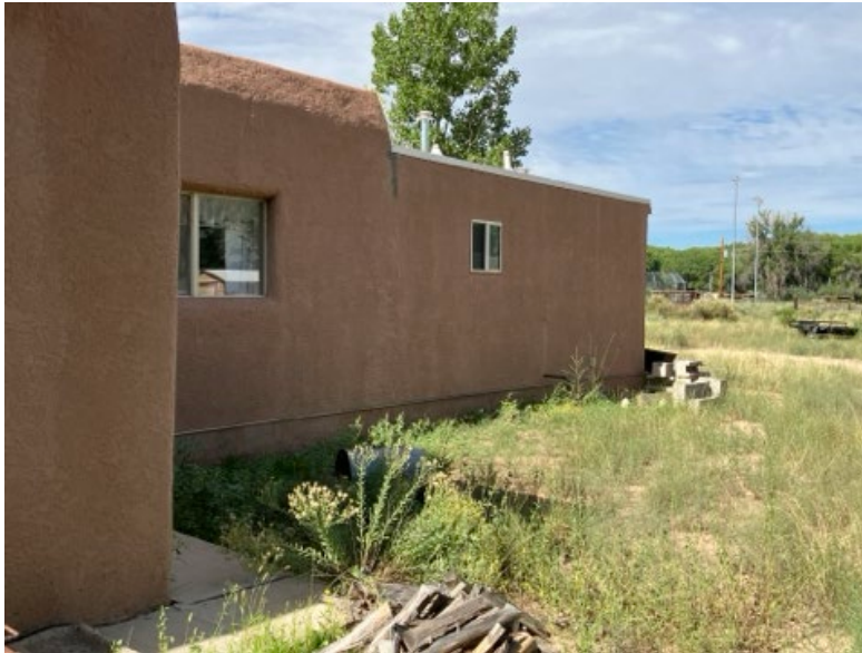
View of the existing sewer service line (SSL) cleanout at the northwest corner of the house. The new SSL will connect to the house at the same location.
