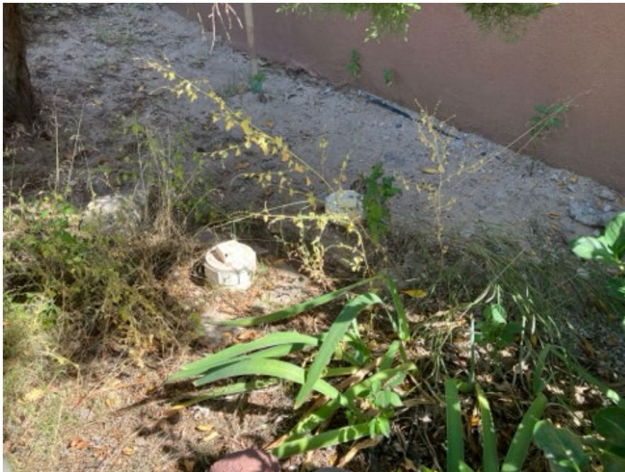
View of the existing sewer service line (SSL) cleanout at the west wall of the house. The new SSL will connect to the house at the same location.
